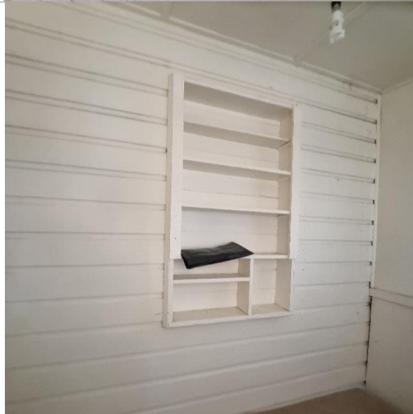
Window opening on southern side of enclosed verandah which can be reinstated. Original chamferboard cladding.
